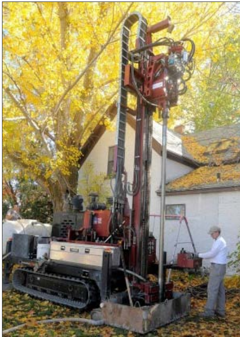
Dewayne Dean drills a hole to install geothermal heating at the home of Anne Hedrich on Nov. 4, 2010. (Eli Lucero/Herald Journal)
